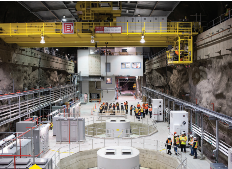
SNC-Lavalin's award-winning John Hart Generating Replacement Project, an innovative underground power station in Campbell River, Vancouver Island.
