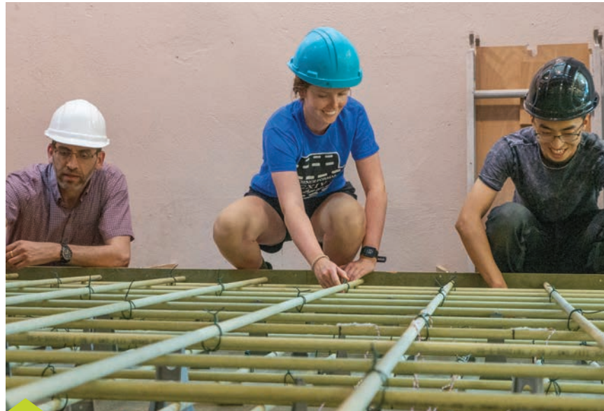
Laura Tauskela, EIT (centre), ties GFRP bars, along with Amir Fam, PhD, P.Eng. (left), and Fam’s current graduate student, Severus Gao, on a bridge that Tauskela helped to design and construct to test ROLLS.
