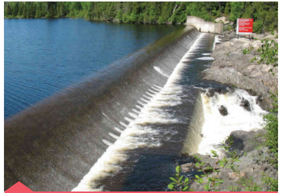
Hatch and FHR Inc. are a Canadian Consulting Engineering Awards winner for the project for reducing life safety risks to the Kashechewan First Nation Community, near James Bay, Ontario.
