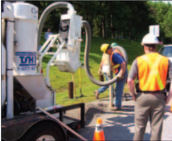
Technicians install test holes on an existing water main in Niagara-on-the-Lake, Ontario.
