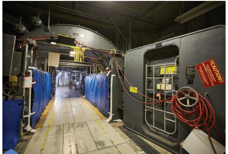
The refurbishment of Darlington's Unit 3 nuclear generator. Jothi Bavan, P.Eng., leads teams of the Darlington refurbishment supply chain. Photo: Ontario Power Generation
